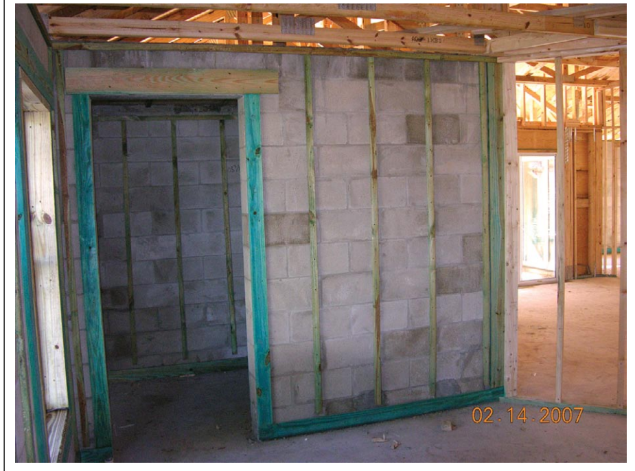
View of an in-residence shelter under construction. Steel reinforced and fully grouted CMU surround the shelter space (New Smyrna Beach, FL).
