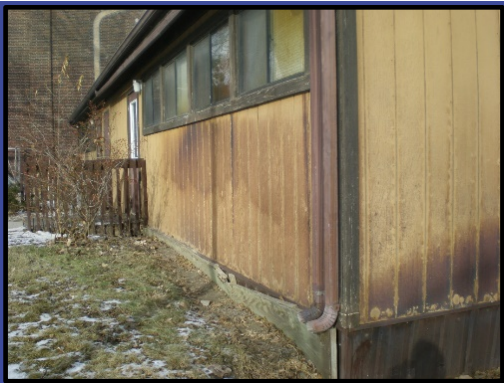
A portable Learning Center in visibly poor condition, with damaged walls, gutters, roof, and window treatments.
