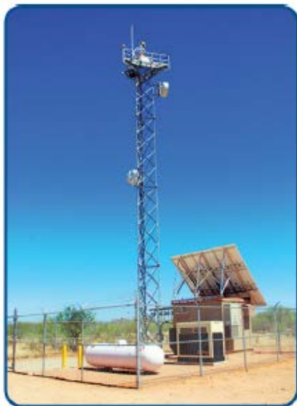
Figure 1. Integrated Fixed Tower 81
