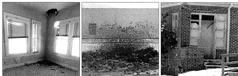
Interior damage of Kerrville Medical Center.
