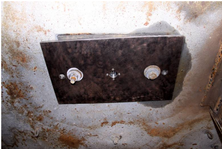
Figure 7a, actual fiber optic front end interface secured on metal mounting plate in ceiling of structure.
