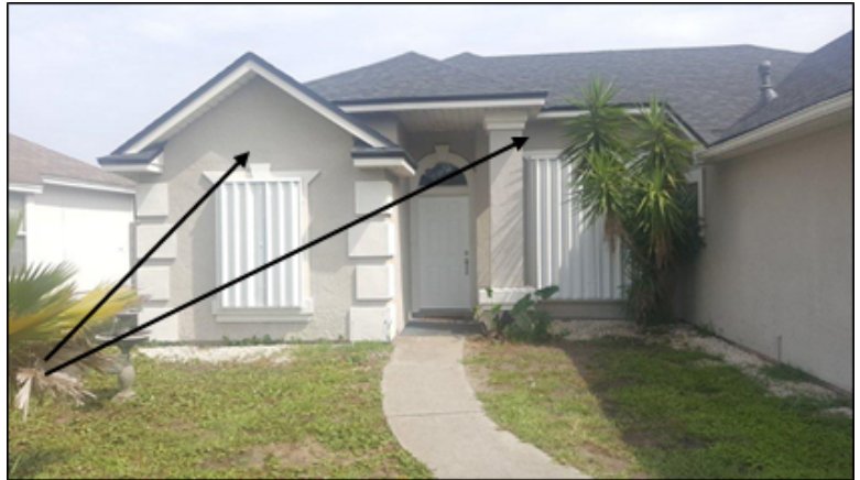
Using the Florida Building Code as a standard for retrofitting, the Florida Division of Emergency Management’s Hurricane Loss Mitigation Program has funded hazard-mitigation upgrades and wind-mitigation projects for residents. Photo courtesy of FDEM.
