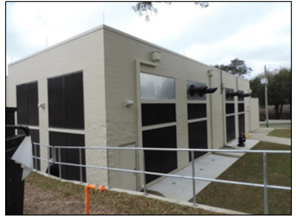
The masonry building provides shelter for the 2 MW generator. Photo courtesy of Florida Division of Emergency Management
