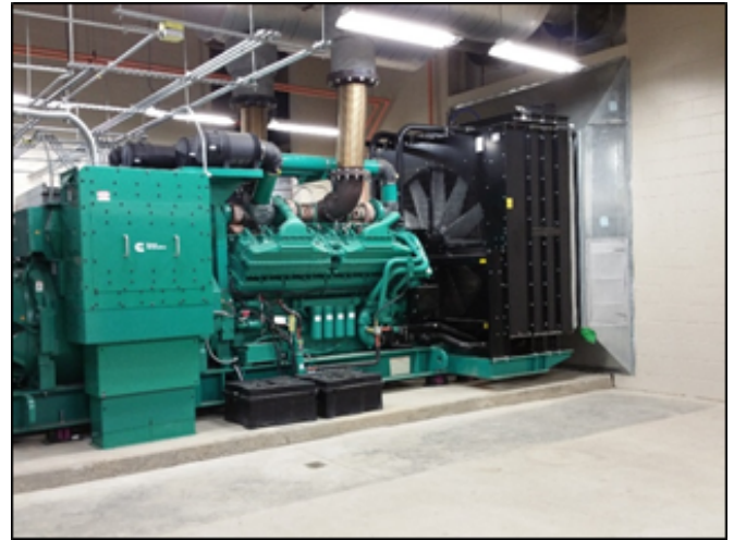
The hospital received a grant to purchase and install this 2MW generator. The generator provides additional power so that non-critical patient care areas of the hospital can be used and not evacuated during a power outage. Photo courtesy of Florida Division of Emergency Management
