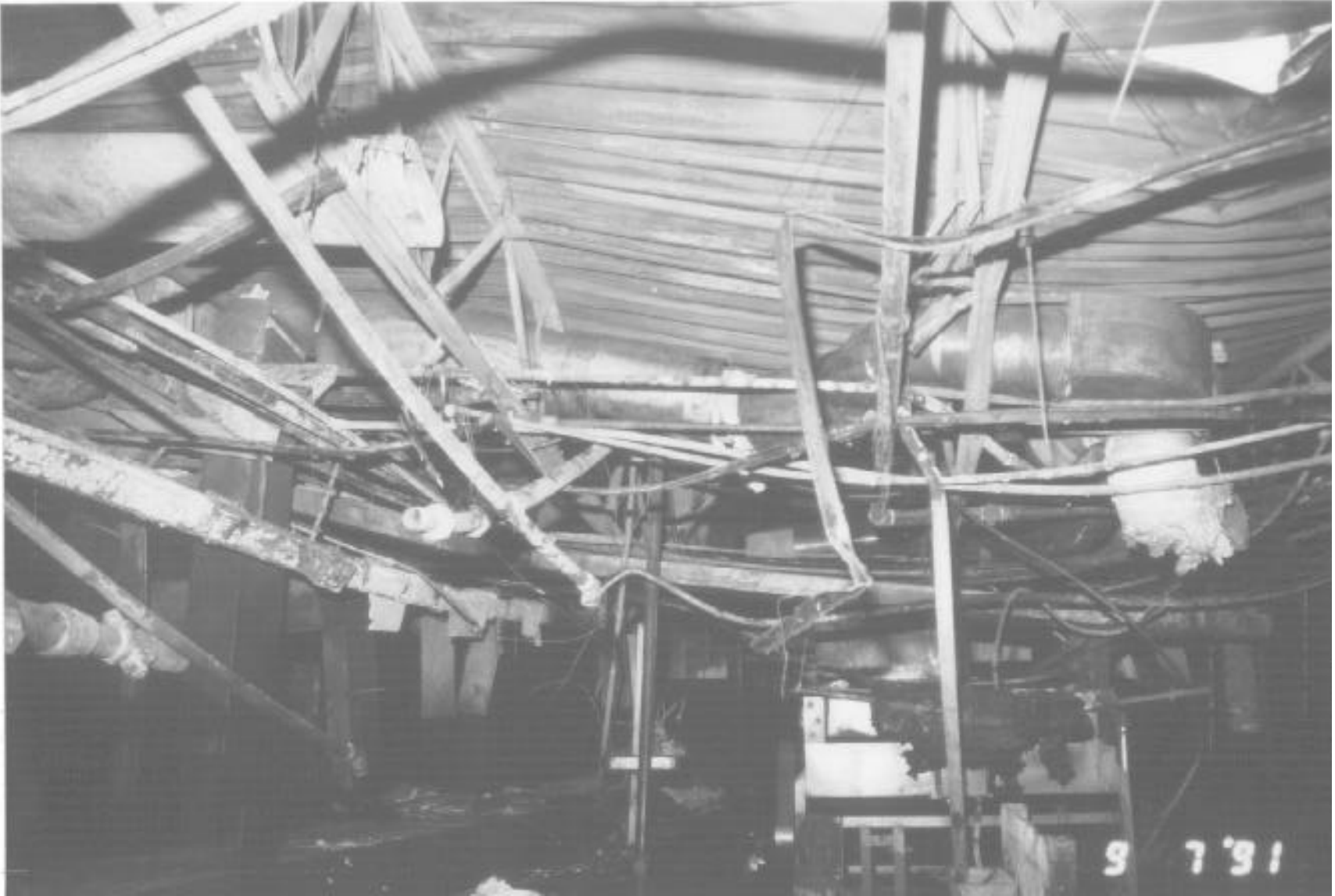
Damage to the steel girders and roof supports over the area of origin.
