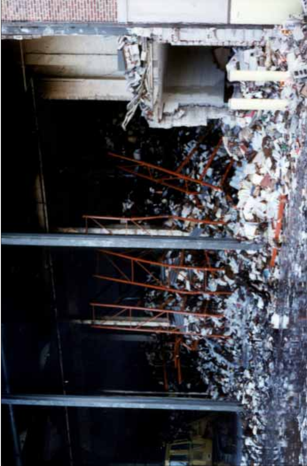
2. Typical of the rack collapse, record box failure, and documents filling the aisles. The brick-faced, hollow concrete block front wall was removed on the night of the fire.
