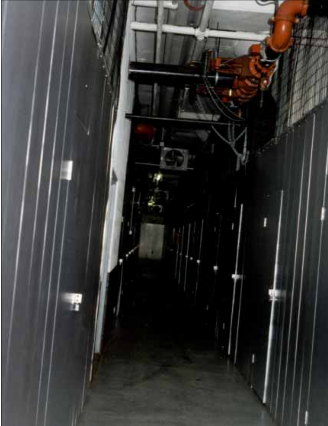
9. Typical public storage rooms or lockers located on the floor above the fire. Note the automatic sprinkler control valves and flow switch located at the ceiling level and the eight feet high solid walls topped by heavy wire mesh.
