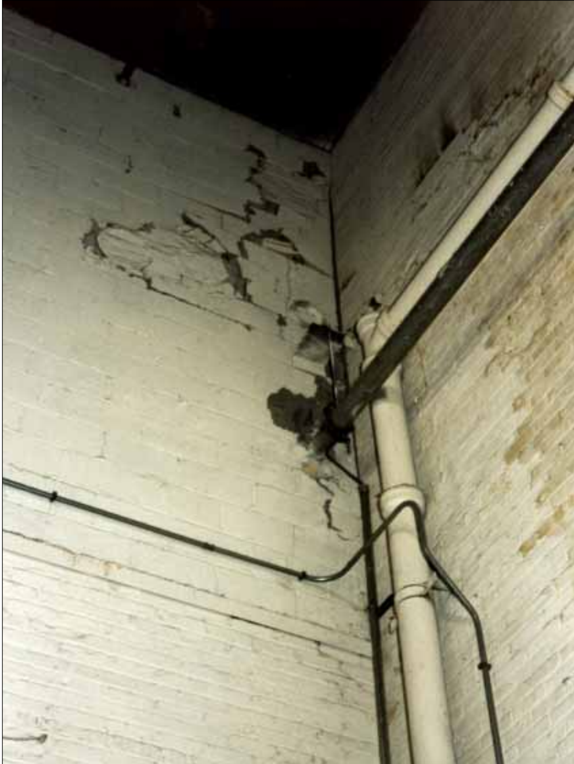
7. Masonary wall damage in Building II, north of the fire building, due to expansion of the fire wall between buildings. This corner is the southeast corner of Space 6.
