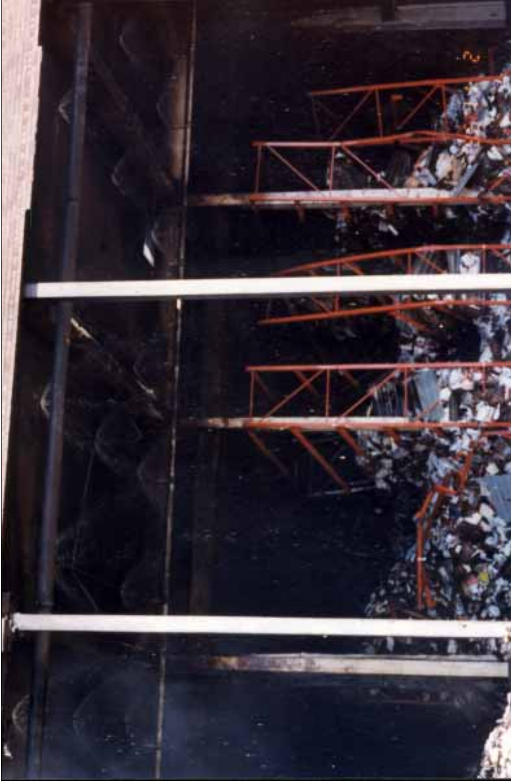
3. Racks and operating overhead automatic sprinklers near the northwest corner of Building III. Complete and partial collapse of the storage racks, shelves, and contents.
