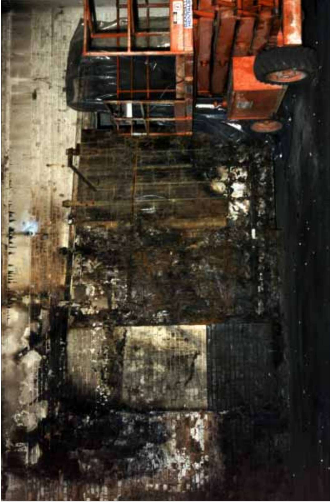
8. The fire side of the metal clad sliding fire door between Buildings III and IV. This door was supported by fire companies operating from the non-fire side of the door.
