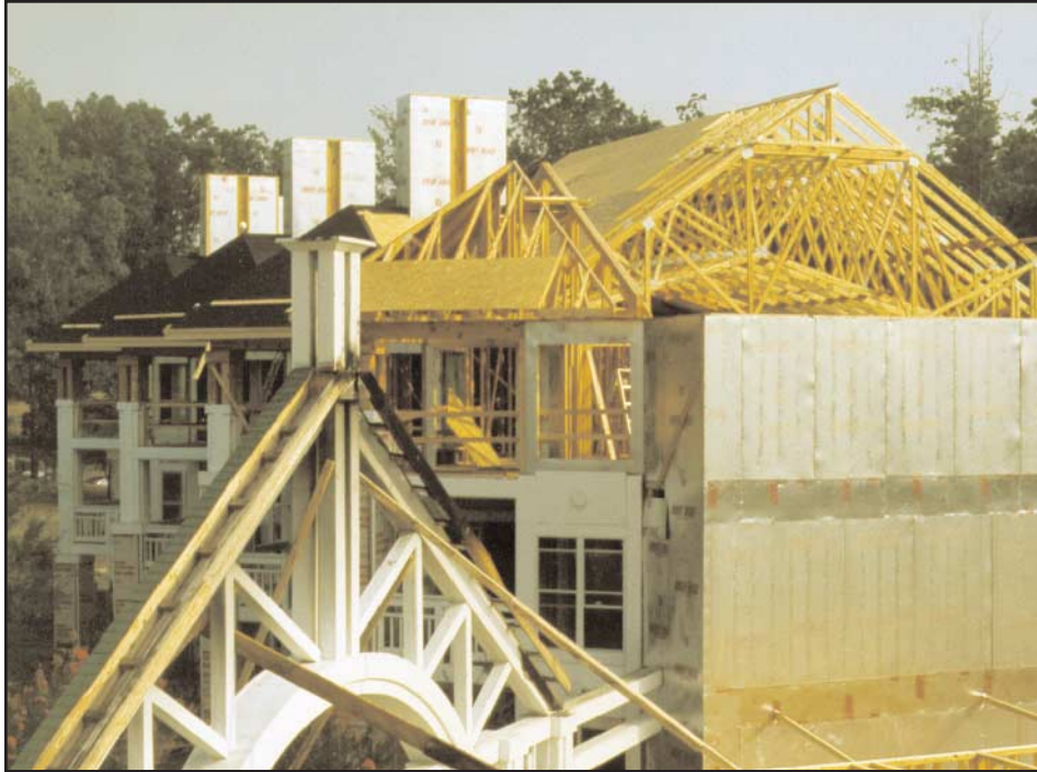
7. The remains of the front archway and the repairs and reconstruction underway for the wing in Photograph 6. The attic trusses and exterior sheathing materials are illustrated.
