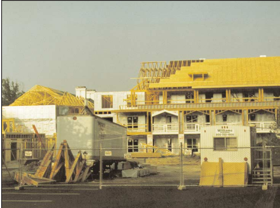
8. Reconstruction underway in Sector B, which is on the south side of the building. The exterior walkways were on this side of the wings.
