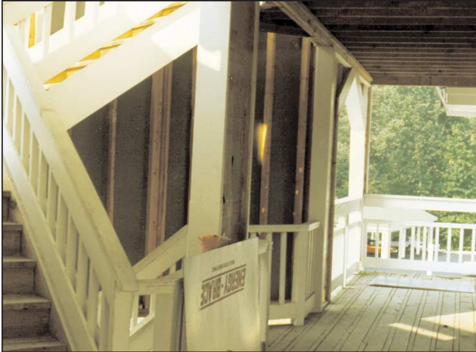
10. The stairway and exterior walkways used throughout the building. Note the gaps in the walkway to allow water to drain and the piece of thin exterior sheathing leaning against the stairway.
