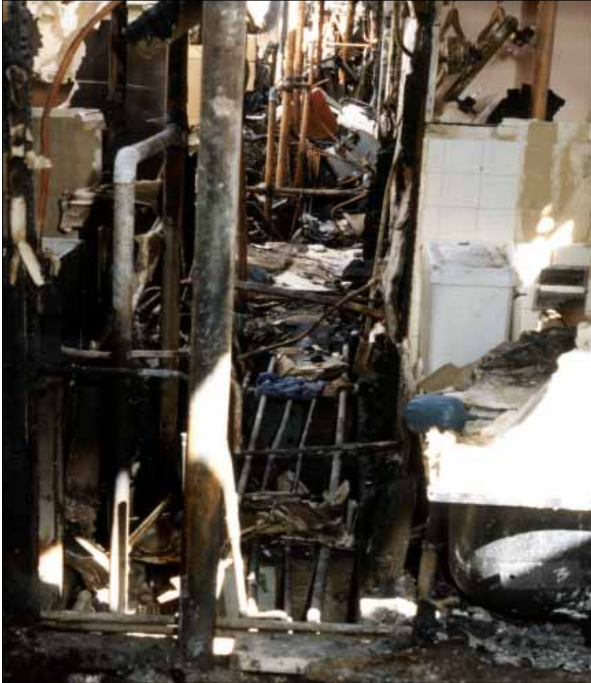
7. The west end of the utility chase in the front wing. Room 222 is to the left and Room 211 to the right. The second floor utility chase walls were burned away.
