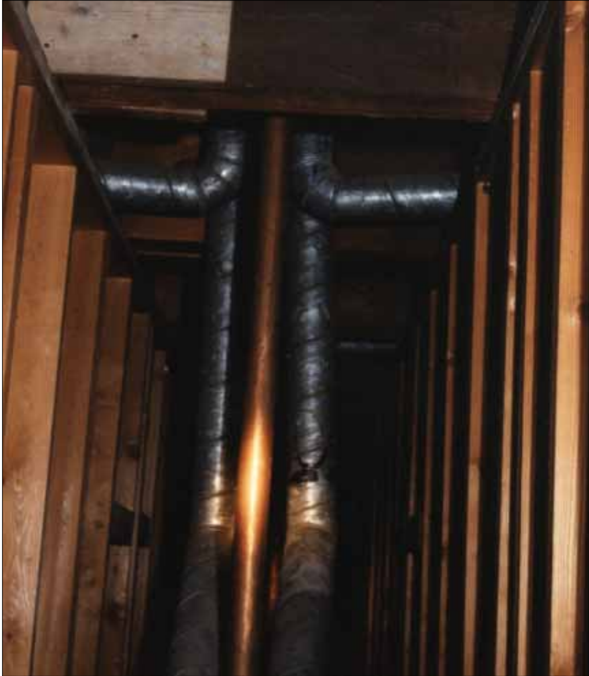
5. The interior of the utility chase between rooms showing the second floor wall construction and the wood beams supporting the roof.
