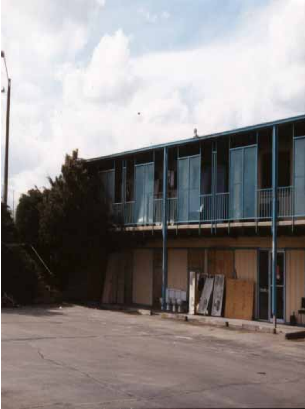
1. Southwest corner of the front wing looking northwest. The 100 level commercial and offices and the 200 level guest rooms are shown. The pine tree shields the entrance to the stairway and storage closet which was the point of origin.
