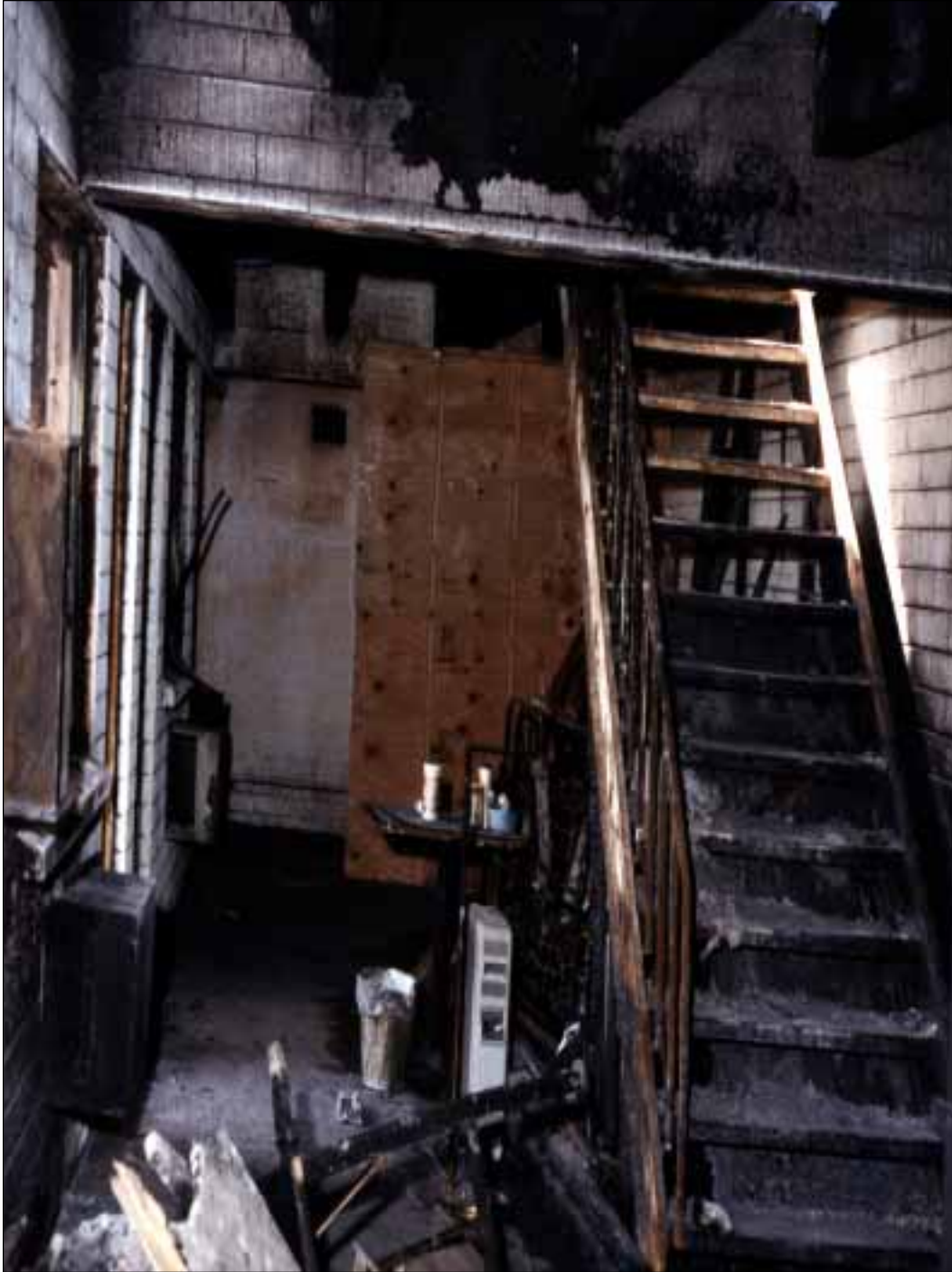
8. The 200 level breezeway area outside of Rooms 220 to 222 looking west. The open stairway to the 300 level is on the right. Under the stairs is another storage room whose wood stud and gypsum board walls were destroyed by the fire.
