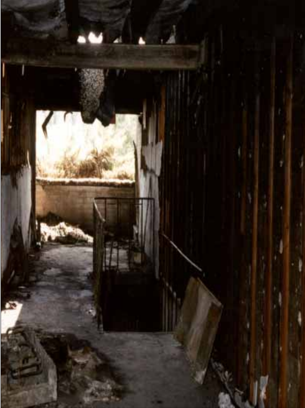
11. The top of the open stairway from the 100 level looking south. A glass in aluminum frame wall enclosed this area just before the partial height brick wall in the background. Room 222 is to the left.
