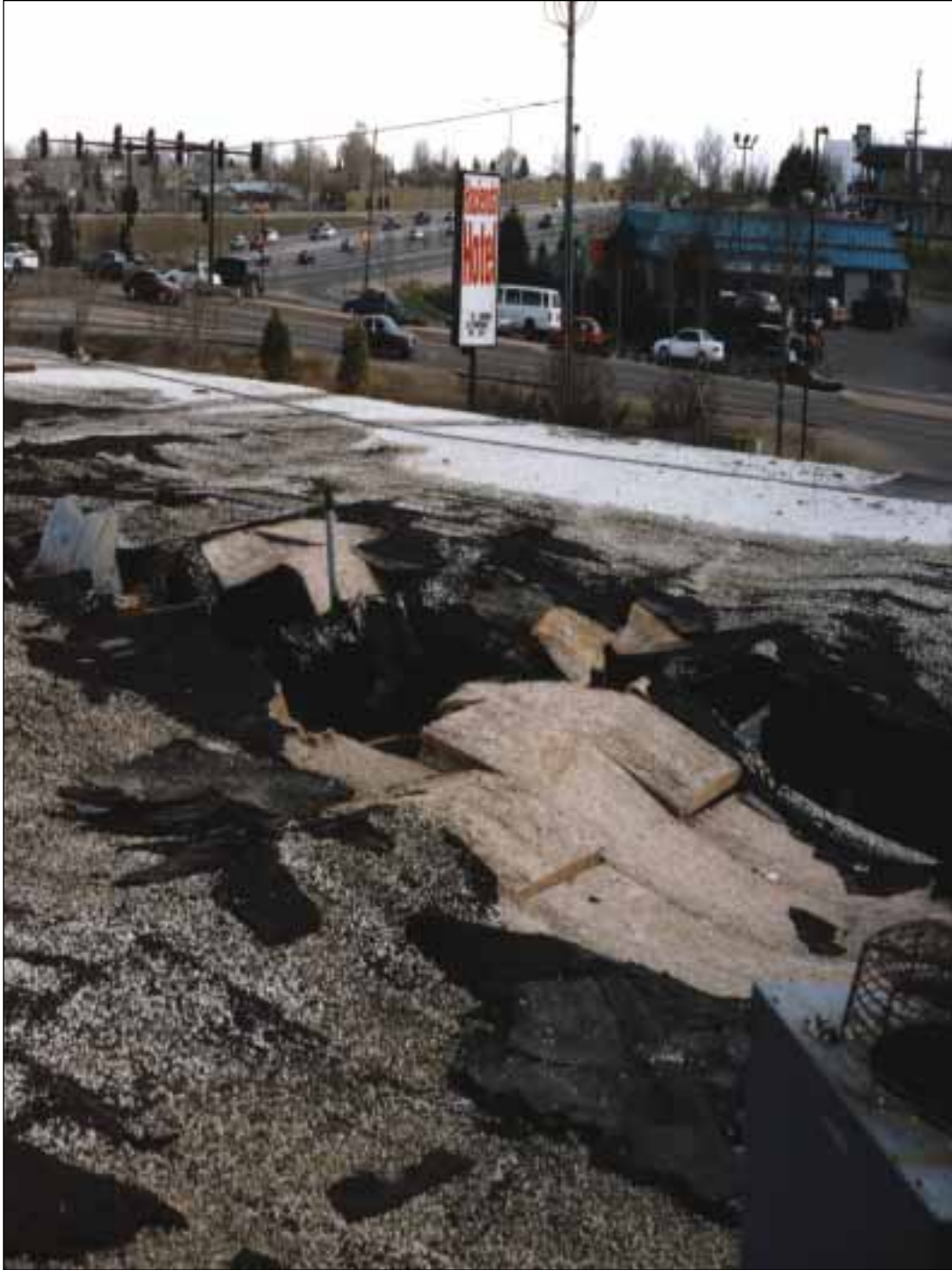
6. Roof over the front wing. The collapsed area is above the utility chase. The roof construction of Tectum board, built-up roofing, and gravel topping is illustrated.
