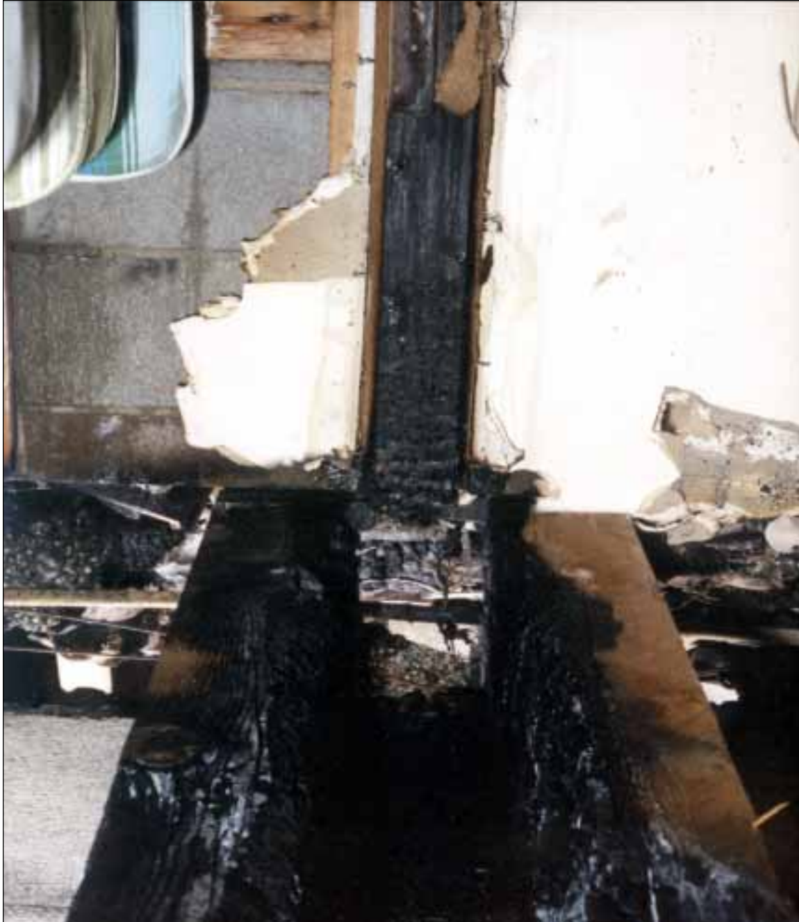
9. A separation wall between 100 level guest rooms that was burned from the inside out. The parallel wood beams formed the top of the wall and the communication to the utility chase is at the back.
