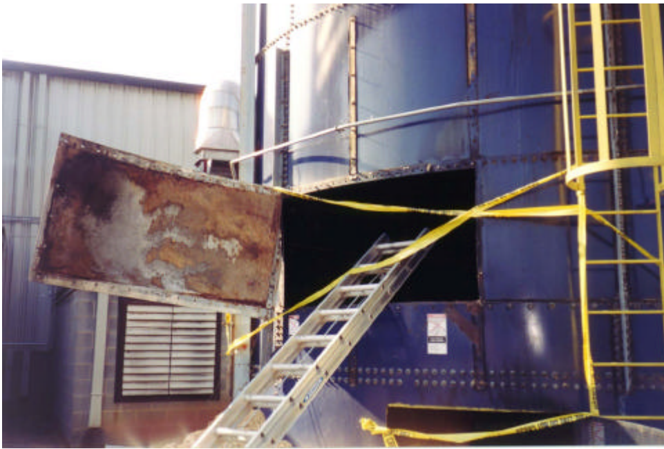
Photo 3. Access plate; area of origin of explosion
