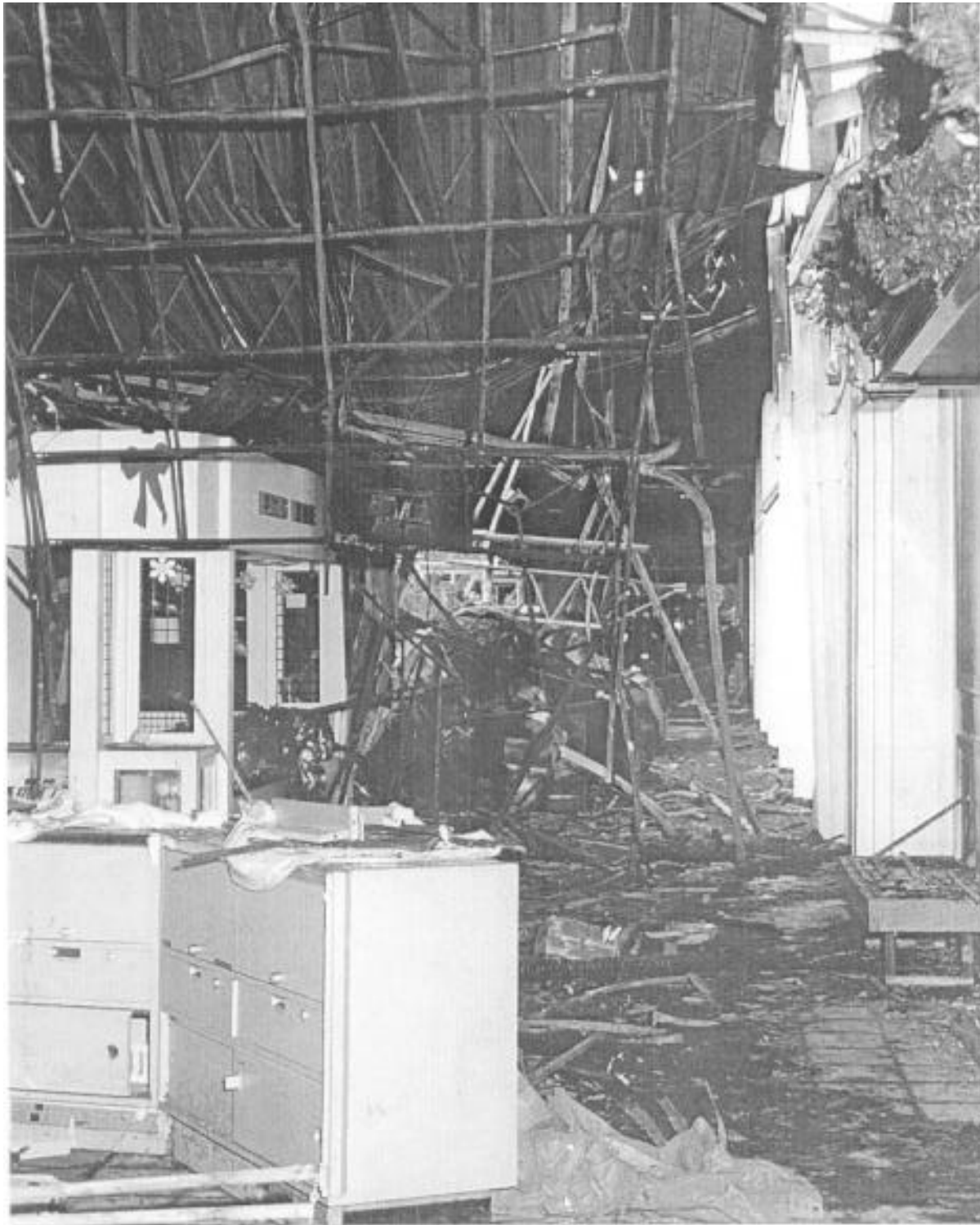
Photograph 6. Moving further east in the covered mall, the counters in the foreground are also in Photograph 3. This area is where the metal roof began a partial collapse. The goods in the kiosks were either stored before the fire or removed prior to the picture.
