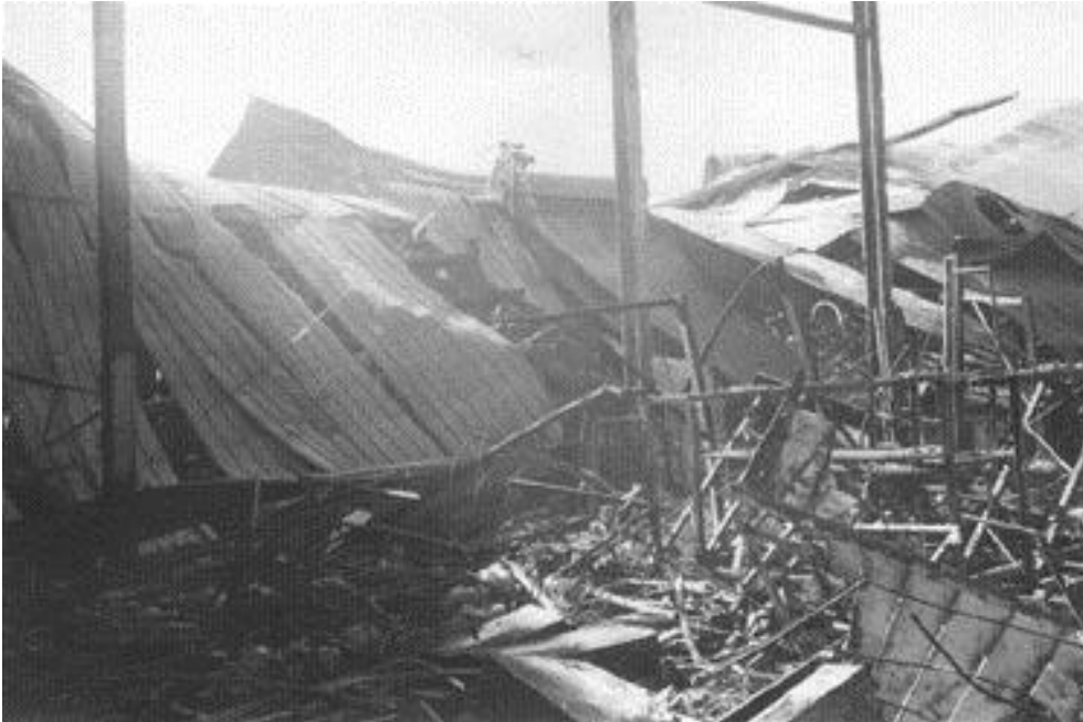
Shows the failure of the rear stage separation wall between the mechanical shops.
