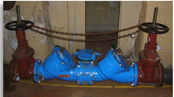
This backflow prevention device may affect the performance of an existing sprinkler system.
