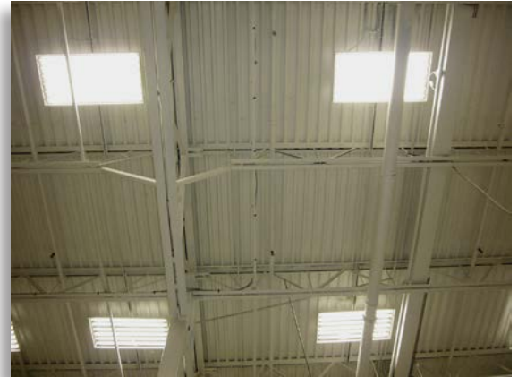
These plastic roof vents are designed to shrink, melt and fall out of their frames to allow smoke and heat to escape.
