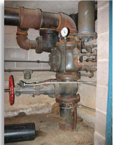
Pipe schedule designs can be employed as part of existing sprinkler systems as long as they meet specific criteria.
