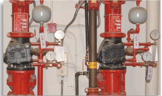
The hydraulic nameplates mounted above the alarm check valves on these wet pipe sprinkler systems are a clear suggestion that these systems are hydraulically designed. (See Coffee Break Training FP-2012-16.)
