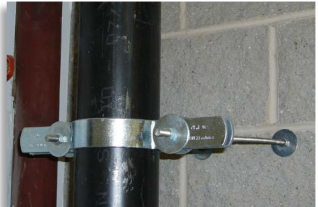
This use of an all-thread rod is a common but incorrect application for sprinkler and standpipe system bracing.
