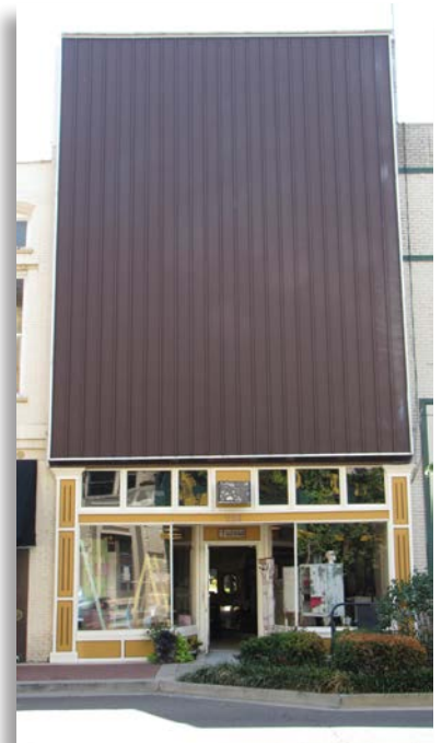
The addition of this noncombustible facade has created a windowless building for the second and third stories of this occupancy.
