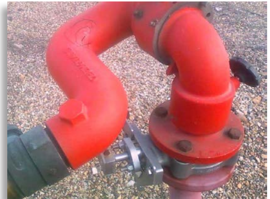
The small crack in the upper left-hand elbow of this monitor nozzle assembly may be a sign of metal fatigue that could lead to a serious operator injury. (Photo/Byron Blake)
