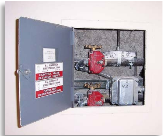
These two supervised, indicating valves control the water supply to sprinklers in the elevator hoistway and machine room of this building.
