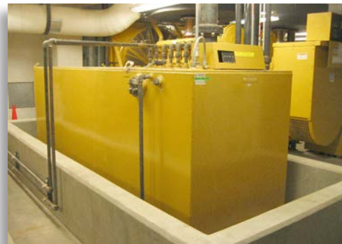
This 1,500-gallon (5,678-liter) fuel tank is sized to fulfill the requirements of a Class 48 emergency power supply system (EPSS).
