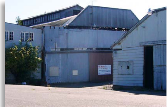
The distance between these Insurance Services Office (ISO) Construction Class 1 buildings influences the Needed Fire Flow (NFF) formula because of the exposure threat.
