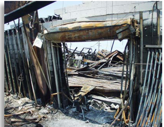
Inadequately protected openings between buildings allow fire and other products of combustion to spread, and they must be considered in the Insurance Services Office (ISO) Needed Fire Flow (NFF) formula.
