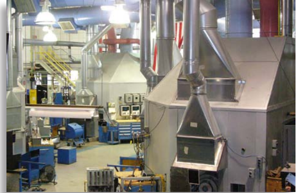
The low combustibility of the operation and contents of this glassmaking facility would enable it to qualify as a Class C-1 occupancy in the Insurance Services Office (ISO) Needed Fire Flow (NFF) formula.
