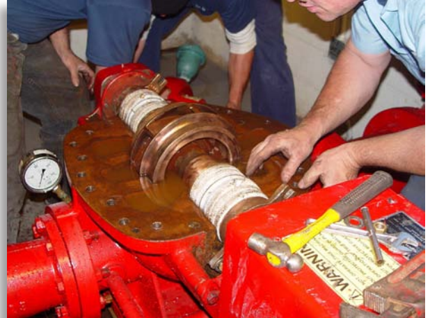
A fire pump service technician inspects the exposed vane for evidence of cavitation. (Photo courtesy of Keith Heckler, Rockville Fire Department, Maryland)
