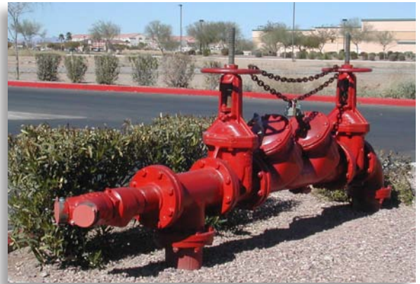
A “code” requires the installation of this backflow prevention assembly; a “standard” describes how it should be installed.
