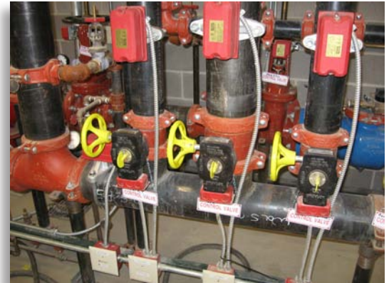
The black pipe on this sprinkler manifold and risers is typical of ductile iron pipe.
