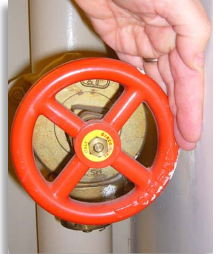
The proximity to the wall of this Class III standpipe hose connection prevents easy access to open or close the valve.
