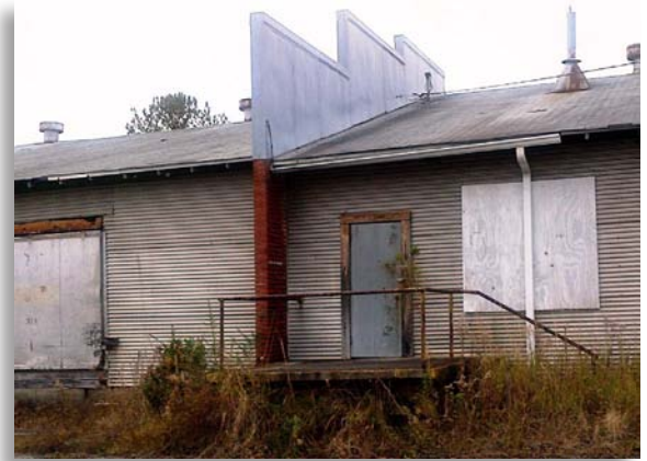
The vertical projection above the roof is the parapet on a masonry fire wall.
