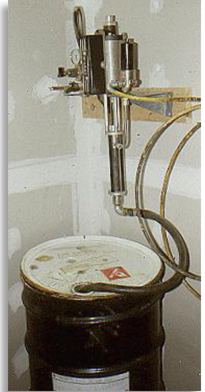
Electrical equipment in the vicinity of flammable vapors must meet specific safety criteria.
