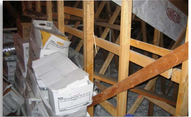
Attic storage like these boxes is prohibited by the fire codes except in specific cases.
