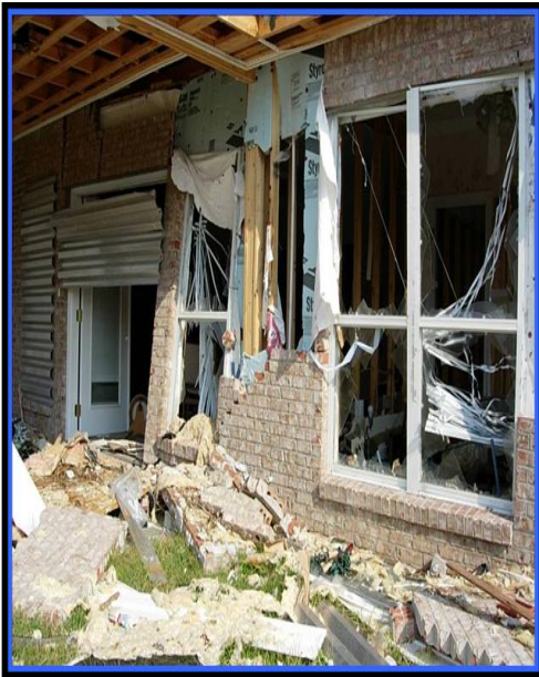
Damaged NPS Facility Photo Courtesy of NPS
