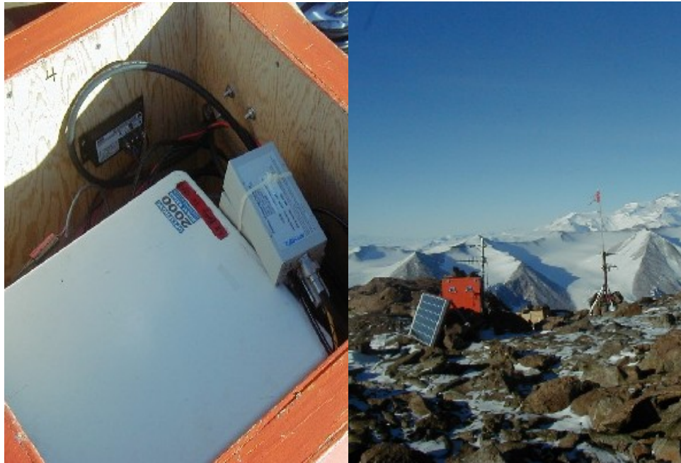
Figure 2.4. Voice and data equipment installed on a mountain top location.
