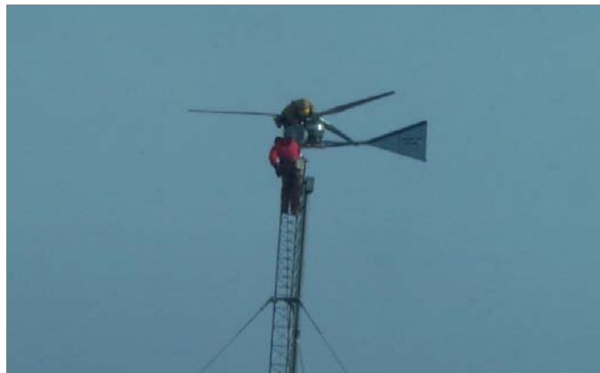
Figure 2.8. HR3 wind generator
