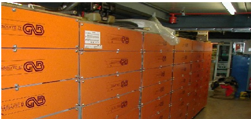
Figure 2.5. Battery bank located at Black Island.
