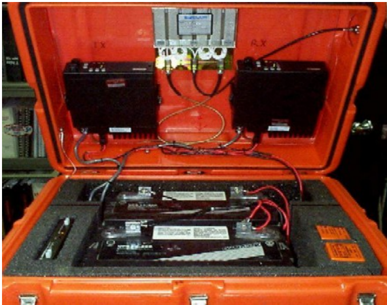
Figure 2.2. Picture of a typical VHF repeater package showing radios, duplexer, repeater controller, batteries, low voltage disconnect, and charge controller.
