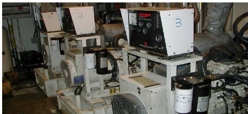
Figure 2.6. Diesel generators located at Black Island.
