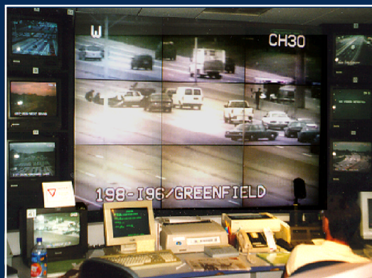
MICHIGAN INTELLIGENT TRANSPORTATION SYSTEMS CONTROL CENTER
