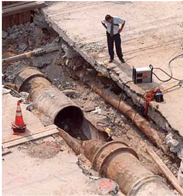
Figure 8. The Water Main Break
