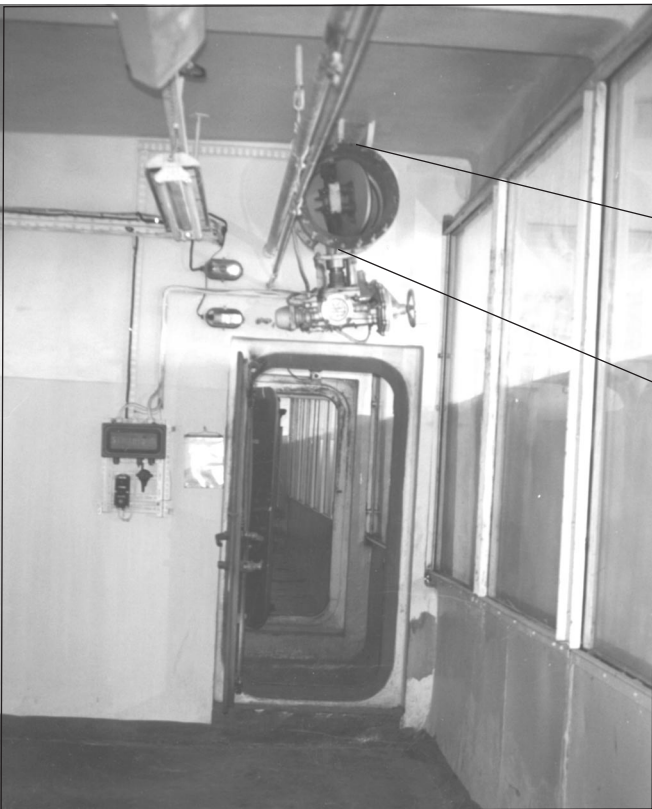
"Butterfly" Airflow Valve Outside a Former Biosafety Containment Laboratory.
