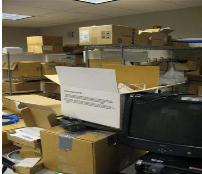
Figure 2: Excess equipment stored in LAN room.
