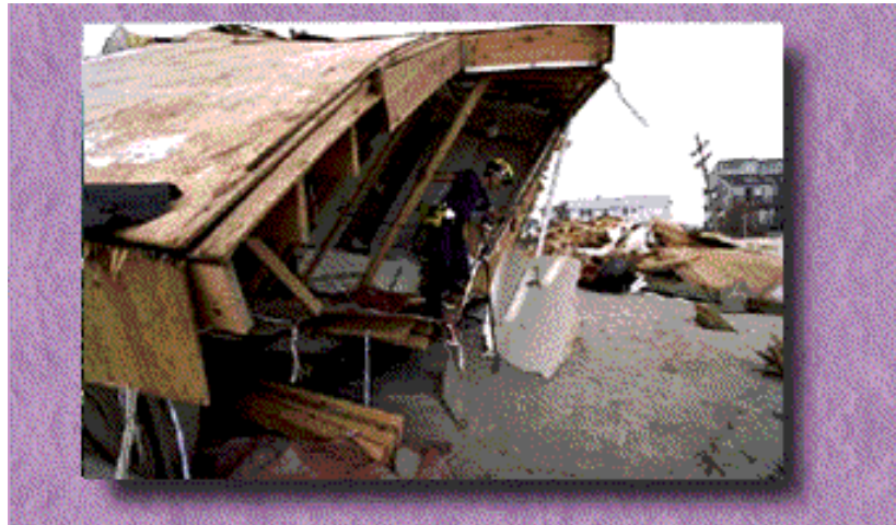
Photo 11. High winds from Hurricane Fran caused most of the damage associated with this storm.
