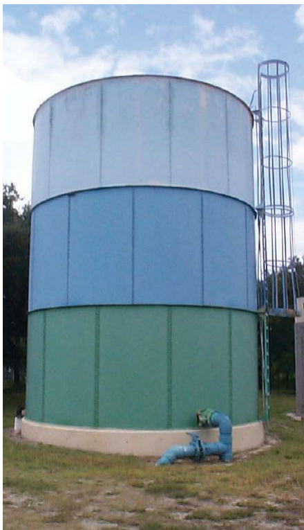
Public access to storage facilities should be restricted
