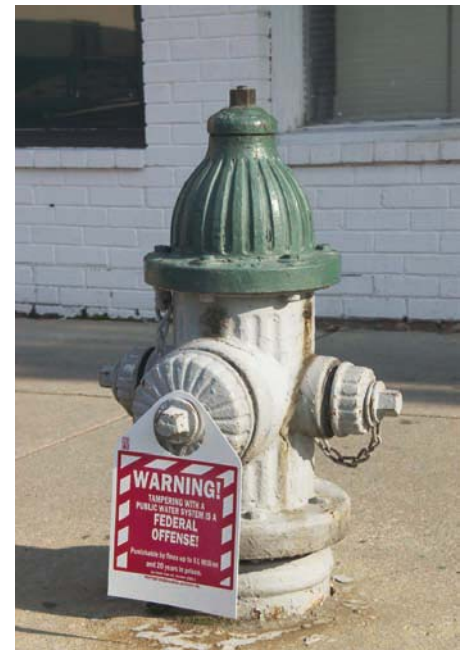
A sign warns against tampering with this hydrant
