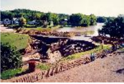
The day after a flood washed out the road over the dam
