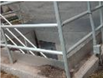
Stairway and lower entrance to anaerobic digester mitigated with cement pad and steel casing
