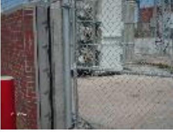
Flood protection wall and stop-log brackets built to protect the main electrical substation
