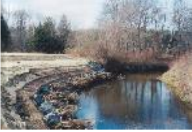
The bioengineered slope along the Mill River shortly after placement in the fall of 2000.
