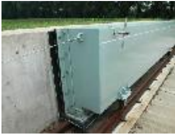
Danville Borough floodwall.
